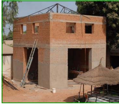
One of the critical stages of waterproofing - adding the plaster that turned water soluble blocks into waterproof walls.
