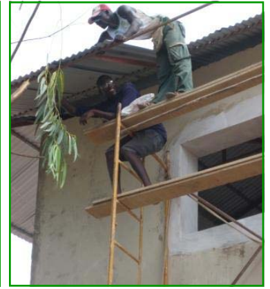
Attaching the sheet metal roof to the second story of the shop.
