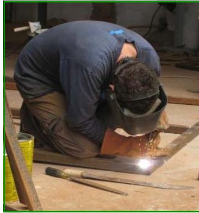
Jason working on the shop doors. Welding in Africa with pants, long sleeves, and protective gear is hot work!
