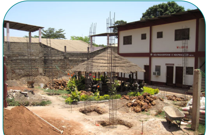
The yard in front of the guest house where the solar system will be. You can see several rebar skeletons that will be cement pillars in a few days
