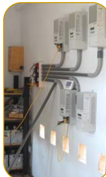
The solar controllers
