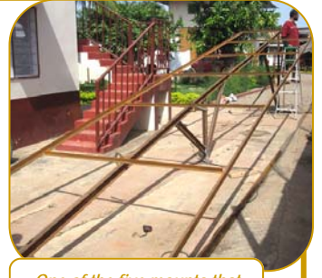
One of the five mounts that will hold six solar panels each
