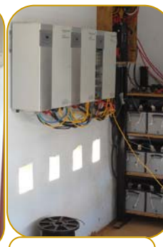
The inverters on the wall inside the controller room
