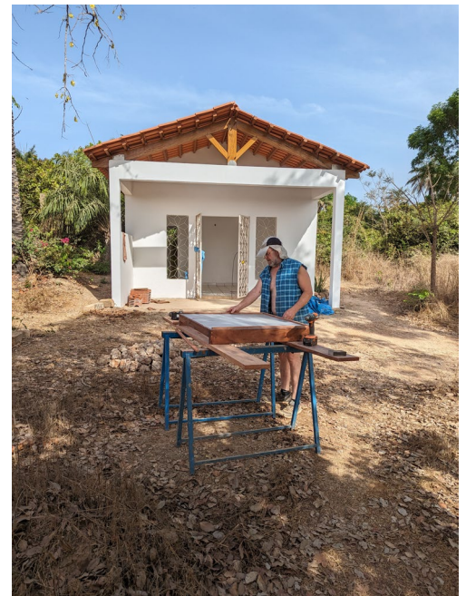
Dad (Paul) screening the windows the Tulsa team made before installing them.
