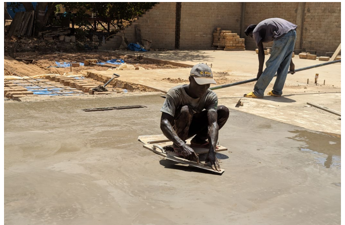
Though not the way it's done around here, my guys have gotten quite good at giving our slab sections a nice smooth steel trowel finish.
