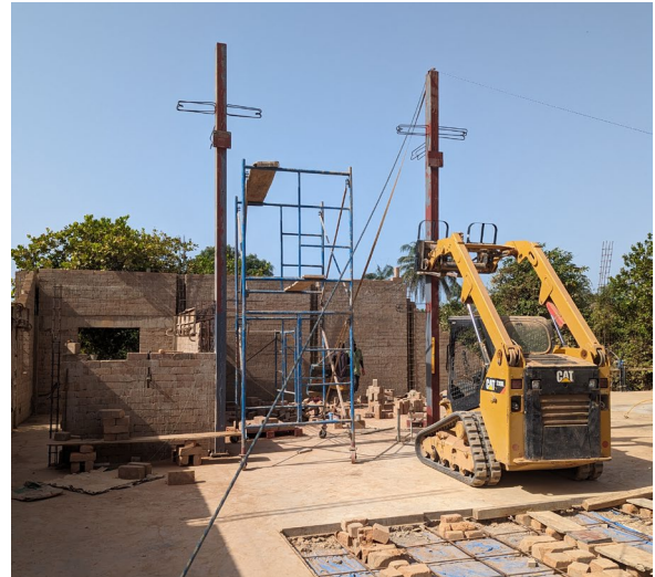
Right: The skid steer has been a giant help in lifting and setting the first pair of steel columns for the new shop!
