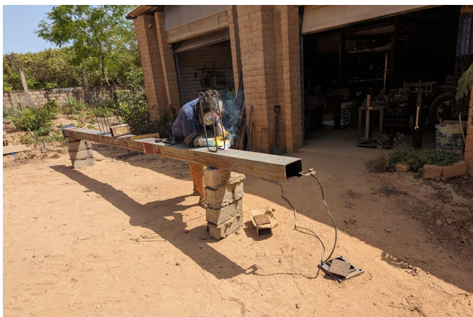
The steel columns were scrap yard finds, now we're welding the attachment points we need onto them before lifting them up.
