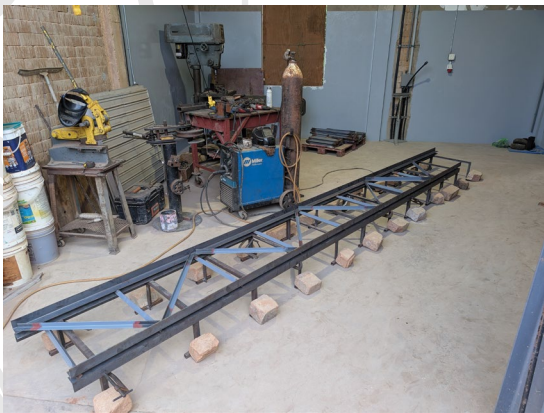
Jigs are key to repeatable work. Time to crank out roof trusses for the central section of the shop!
